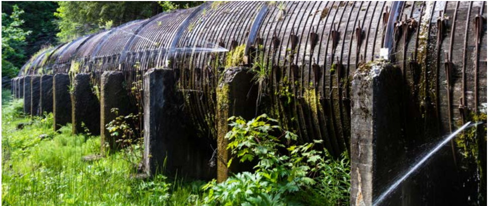
Wooden 12-foot pipeline diverting water from the North Umpqua River, USA, to a powerhouse
